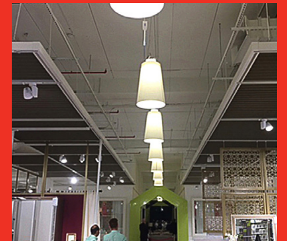
Structural Overhead Power Grid Integrates Electrical and Mechanical elements to support the operations of a store
